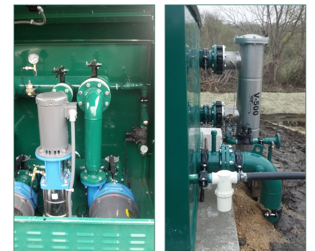
Lift Station Pumps (left) and Filter (right)
